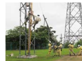
Training to build temporary steel tower with assuming damaged steel tower or breaking of power lines
