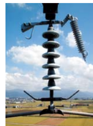
Lightning protection system for transmission line
