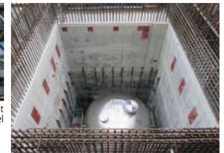
Main body of filtered vent equipment (July 2015)
