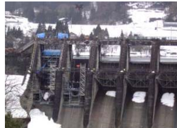
Exchange for maintaining function of spillway gate (Jinzu Daiichi Hydro Power Plant)
